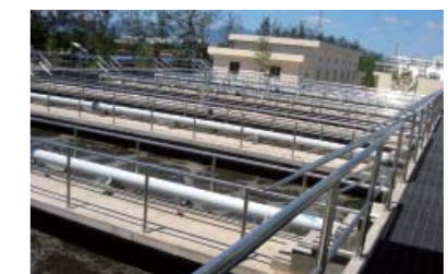
Fig. 2. View of Beijing Miyun MBR plant for municipal wastewater treatment (design capacity: 45,000 m 3 /d)
